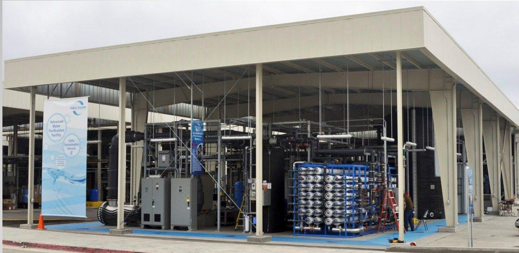
Advanced water facility in north county San Diego (La Jolla). The filtration systems are shown.
